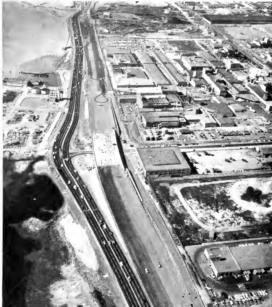
View during construction on Powell Street interchange, which is now nearing completion. Traffic has been routed over a six-lane detour complete with temporary traffic signals during the construction period. Portions of this detour will be retained as a frontage road upon completion of the project.
